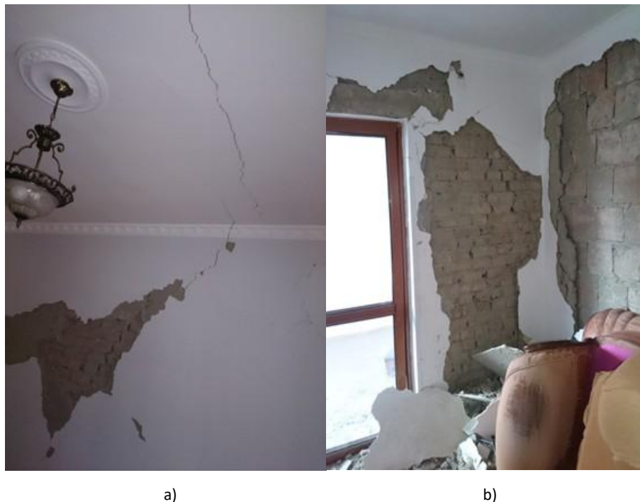
Figure 7. a) Diaphragm-related failures, b) Poor material and substandard workmanship-related failures.
