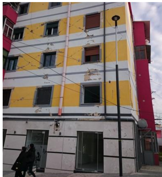
Figure 6. In-plane shear failure of masonry piers.
