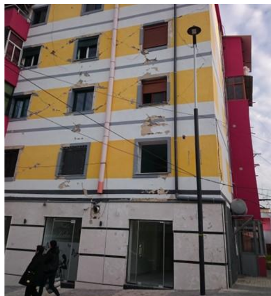
Figure 6. In-plane shear failure of masonry piers.
